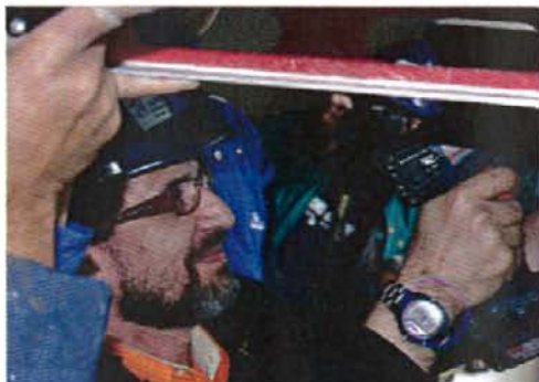
Shaukat, father of partner family, helps install kitchen cabinets in what will soon be his family's new home.
